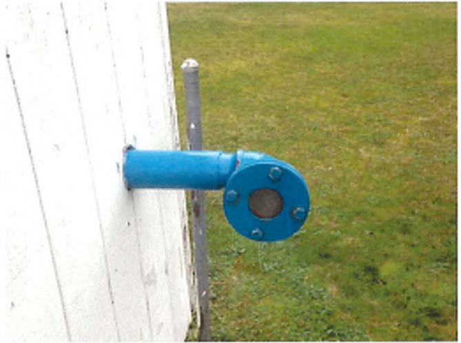
Photograph 10: Well House #2 Pump to Waste Line Does Not Drain to A Splash Pad
