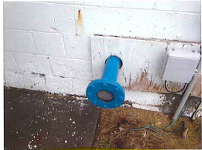
Photograph 6: Well House #1 Pump to Waste Line Does Not Drain to A Splash Pad
