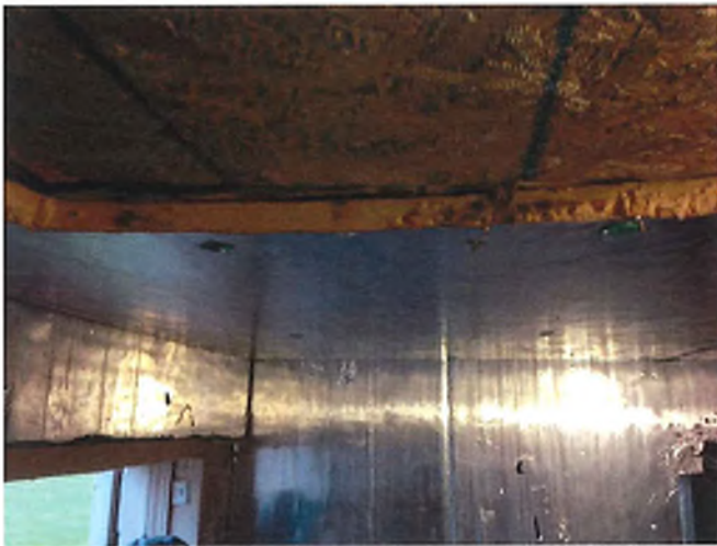
Photograph 9: Well House #1 Roof Leak
