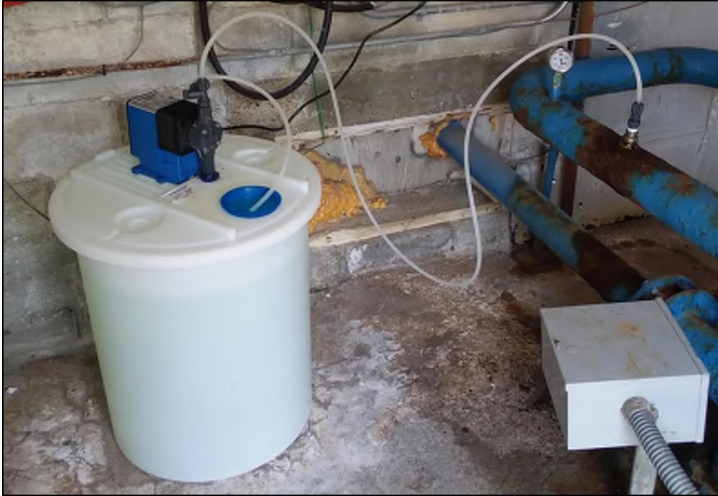
Figure 3-9 Well #1 Sodium Hypochlorite dosing equipment
