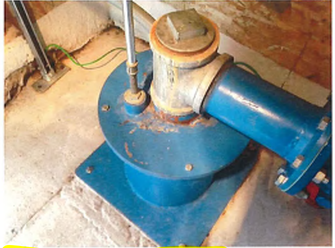
Photograph 8: Well House #2 Well Casing
